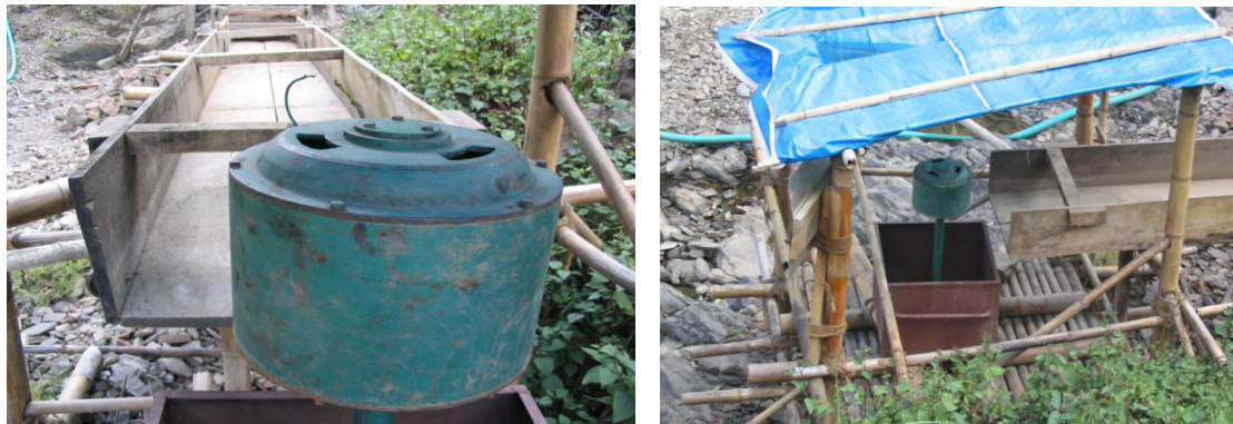
Figure 2.7 Photographs of Pico Hydro power
